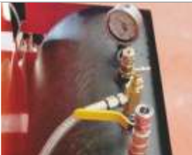
INBUILT AIR COMPRESSOR
