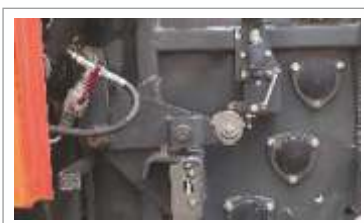
DENSITY CONTROL UNIT
